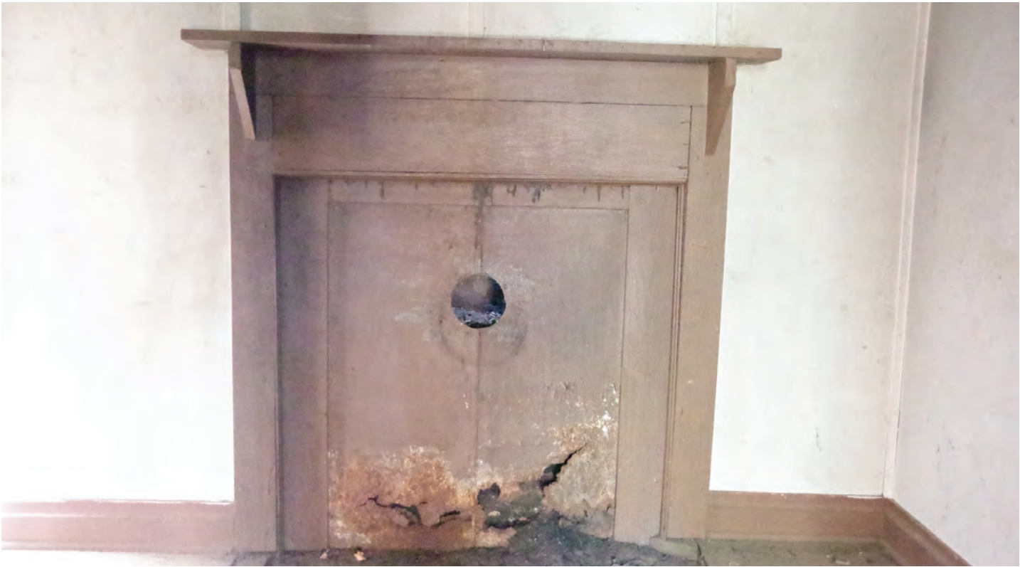
Painted mantel with infill and rustication of metal sheet
