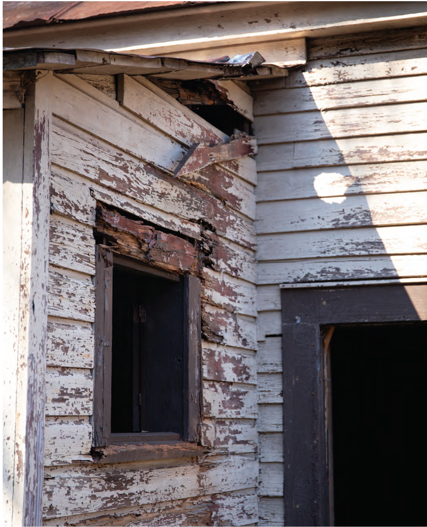
Shed-roof addition, eave and fascia detail, missing sash in addition window opening
